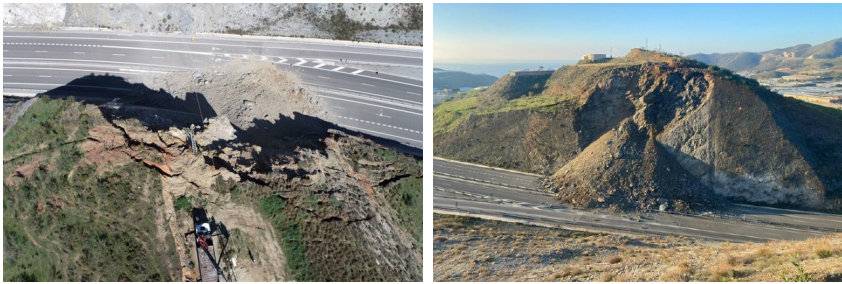
Figure 9: Landslide in Castell de Ferro, A7, Spain, 13/3/2021 (EU Riskcoast _Sudoe project).
